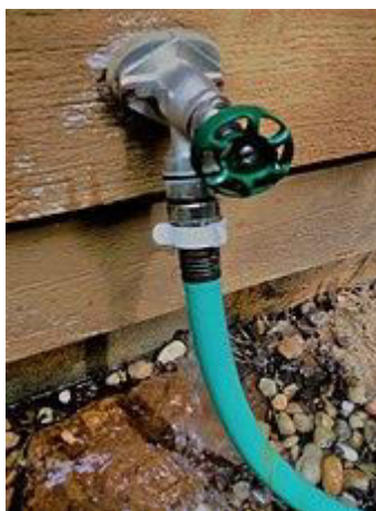
Leaking garden hose bib
