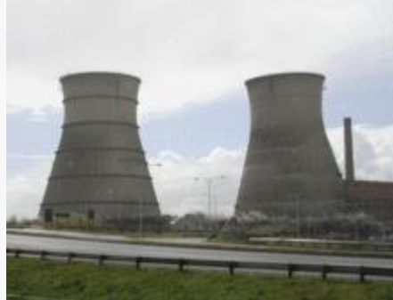
Demolition of the cooling towers of a power station, Athlone, Cape Town, South Africa, 2010
